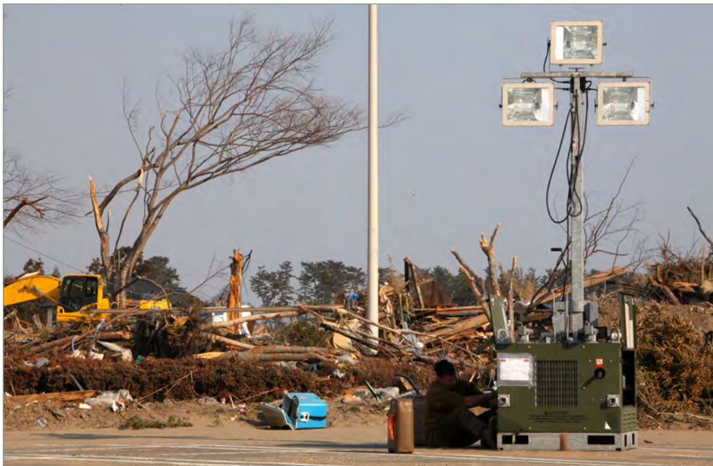
Lance Corporal Robert Branch, an electrician attached to the 3rd Marine Logistics Group, repairs a generator-powered floodlight at the Sendai airport on 29 March 2011. (Gunnery Sgt. J. L. Wright Jr., USMC; DVIDS, 383924)
